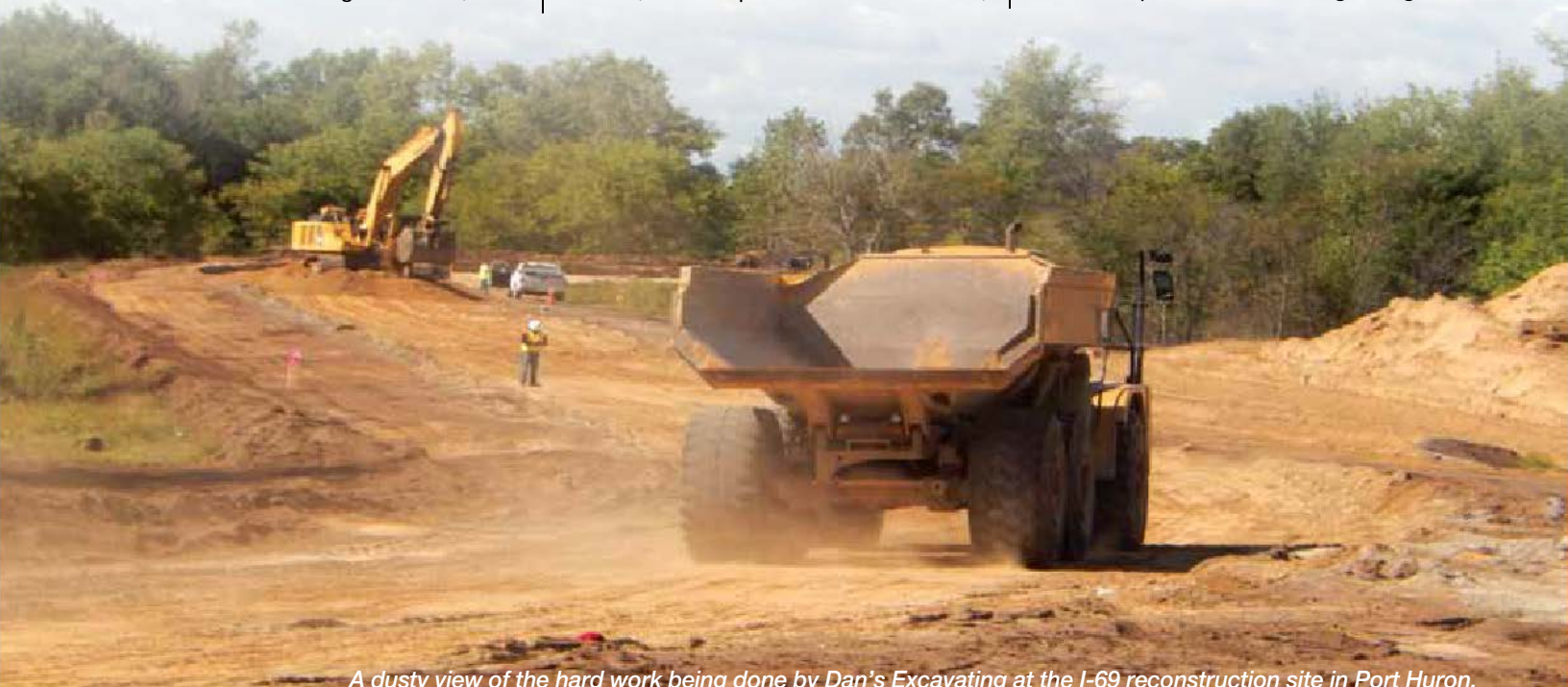
A dusty view of the hard work being done by Dan's Excavating at the I-69 reconstruction site in Port Huron.
