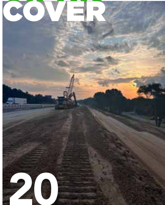
The noise barrier subgrade on the Interstate 94 project in Berrien County. Photo courtesy of Adam Rochefort.
