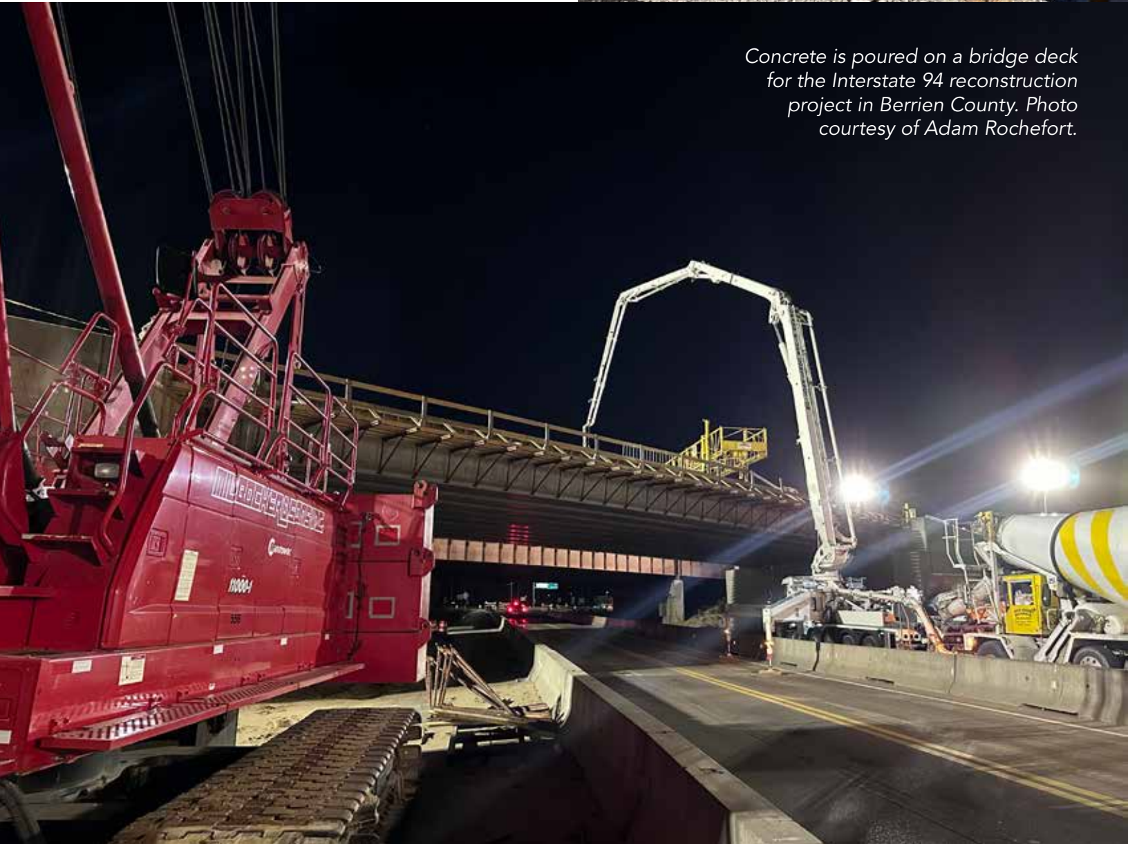
A bridge beam is set on the Interstate 94 reconstruction project in Berrien County. Photo courtesy of Adam Rochefort.
