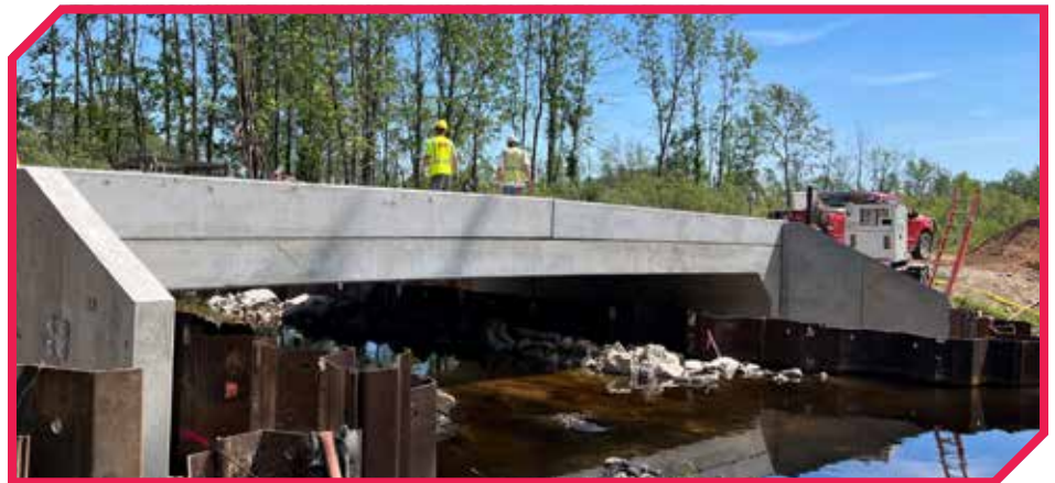
Project Photo: 36'x5' precast/prestressed, three sided, low/span bridge, which was installed in Menominee County in September 2022. The contractor was Bacco Construction Company.
