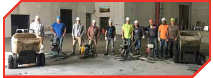
Our concrete crew finishing up the last major floor pour at the Marquette Municipal Service Center in Marquette, Michigan.
