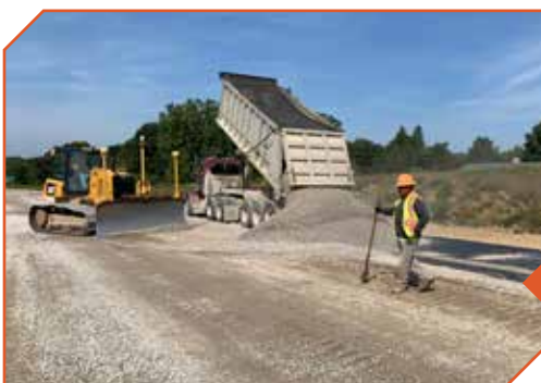
Open-graded aggregate base course is placed on the Interstate 69 project in Lapeer County.
