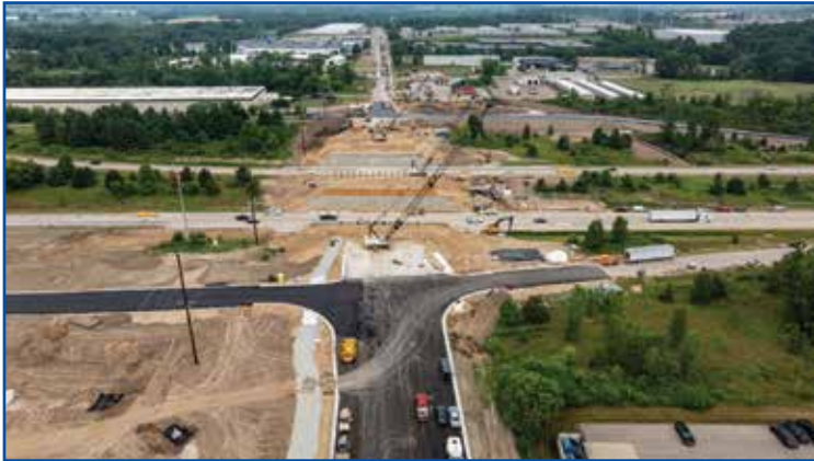
Fruit Ridge Avenue looking north from 3 Mile Road. Eastbound Interstate 96 ramps were realigned. Work to realign the westbound I-96 ramps were close to complete. Photo courtesy of the Michigan Department of Transportation.
