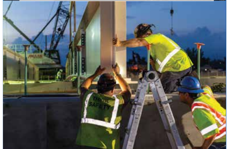
Beam setting for the bridge over westbound Interstate 96 occurred on the night of July 25, 2025. Photo courtesy of the Michigan Department of Transportation.
