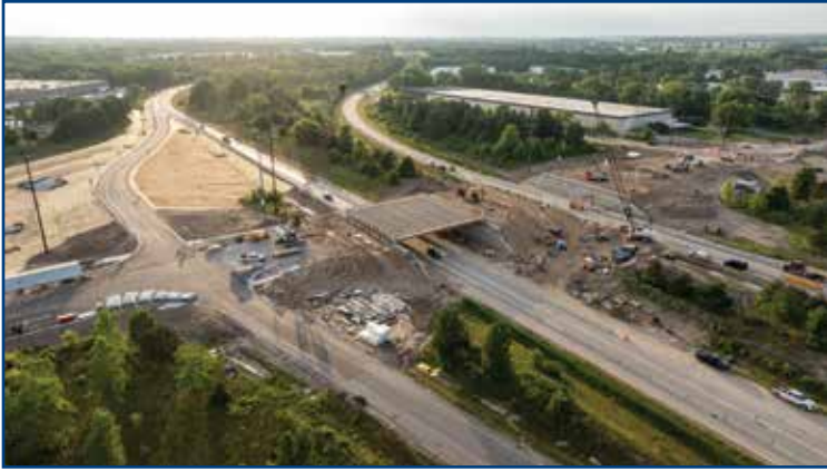
Beams for the bridge over eastbound Interstate 96 were set the weekend of July 18, 2025. Preparation for the westbound bridge beam setting for the weekend of July 25, 2025, followed. Photo courtesy of the Michigan Department of Transportation.
