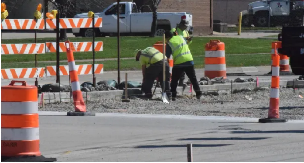
Road-construction workers at Kelly Road 15 Mile Road in Fraser in 2024. MACOMB DAILY FILE PHOTO
